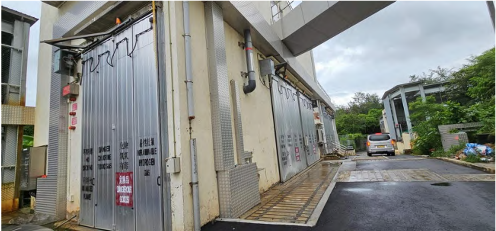
FIGURE 10 Site Photo 5 - Existing On-site Chlorine Generation
