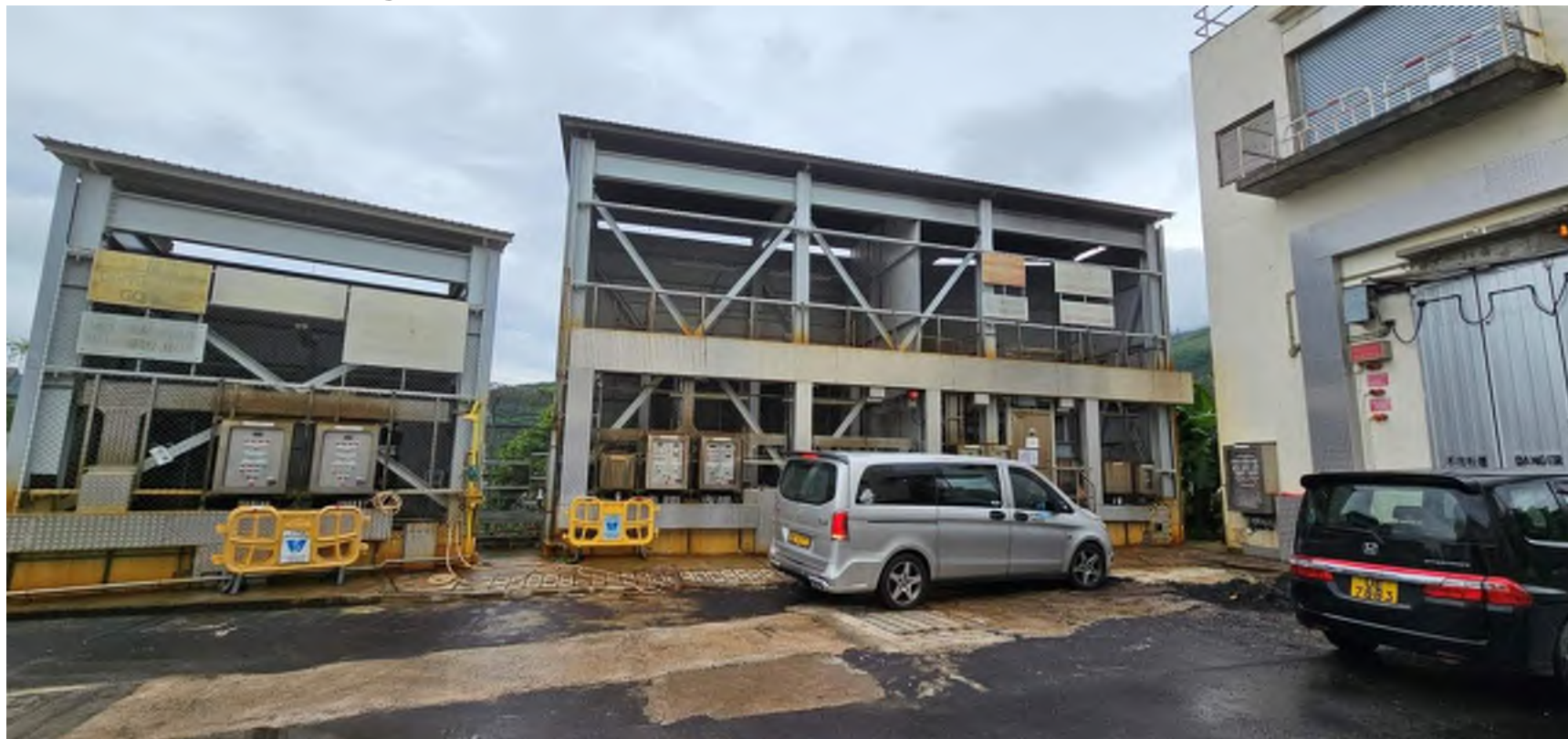
FIGURE 11 Site Photo 6 - Existing On-site Chlorine Generation
